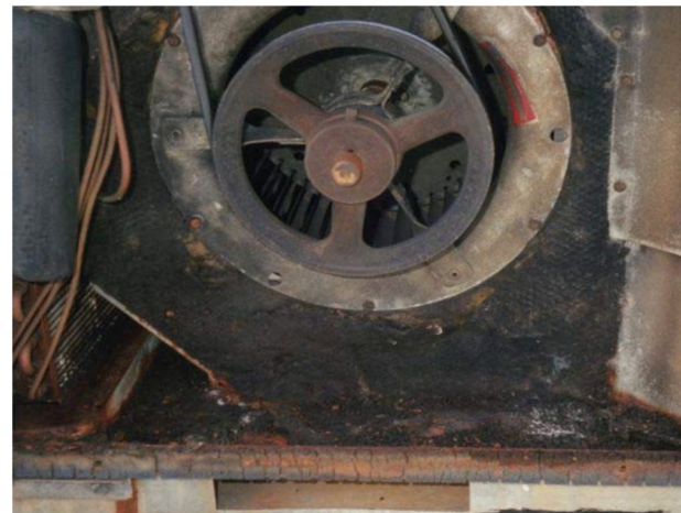
FIGURE 4: While this illustration only shows a flawed air handler, the impact on the health of building occupants can be fully appreciated only when it's realized that all air in a conditioned space passes through the contaminated air handler several times per hour.
