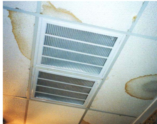
FIGURE 5: A damaged and contaminated ceiling.
