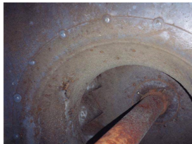
FIGURE 3: A damaged and contaminated air handler.
