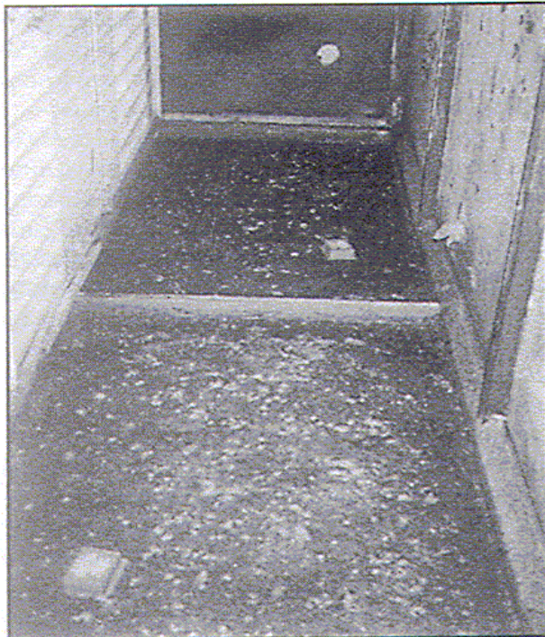
(a) Drain pan - large air handler
