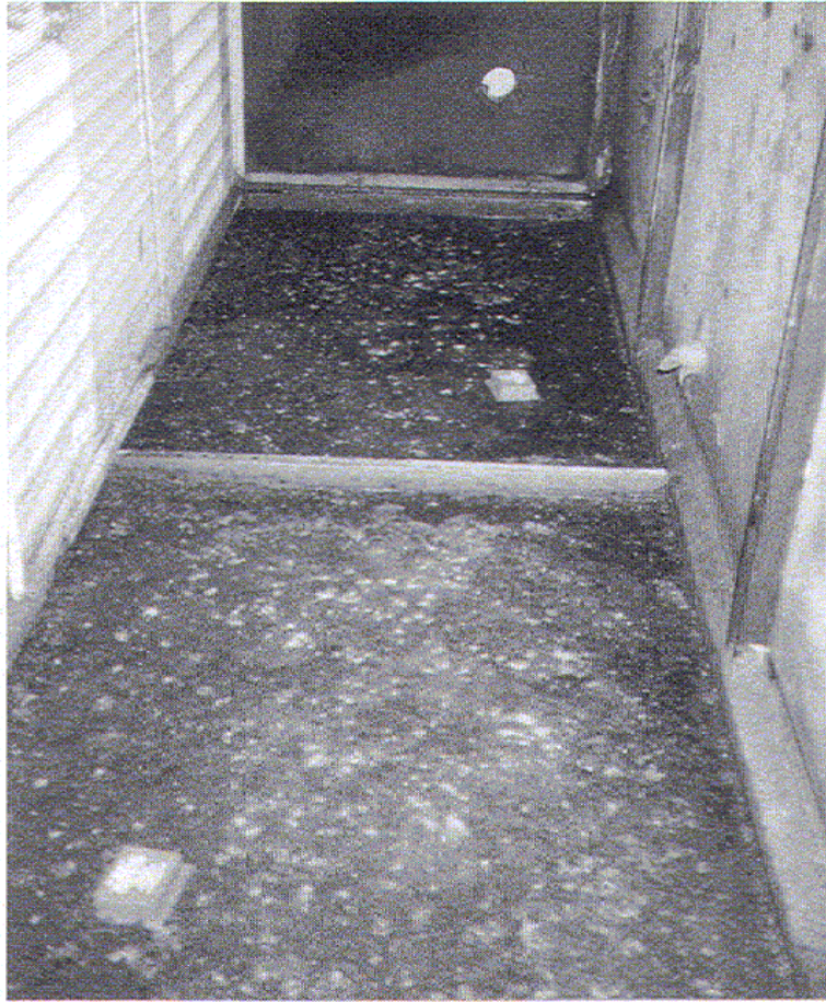
FIGURE 18.8.21 Photo showing contamination in wide drain pan.
