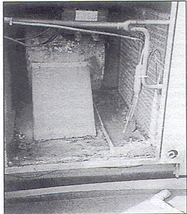
(b) Drain pan - packaged hvac unit
