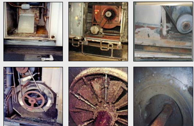
Figure 2. Damaged and health threatening air handlers caused by failed drain systems
